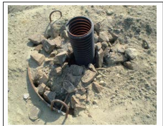
Picture 3-9 Gas venting facility that is in the process of being plugged and buried (bad example)
